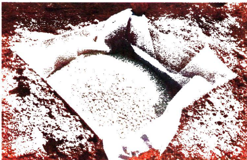
Fig. 5. Sandy Gravel is deposited into the pit box up to the ground level
