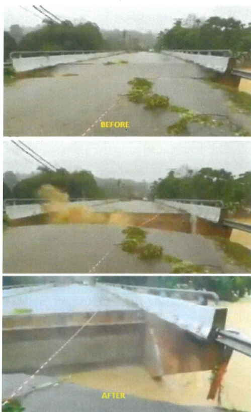
FIGURE 6. Bridge collapse in Raub, Pahang in January 2021 due to high discharge of river and extensive scour around pier and abutment.
