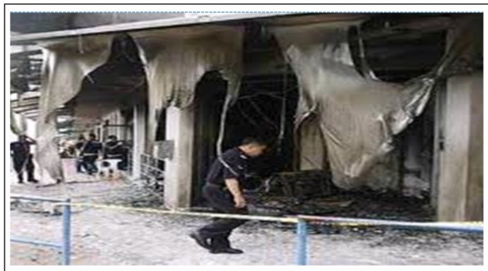
Figure 1.2: Damaged due to the attack on the building (Mazwin, 2010).
